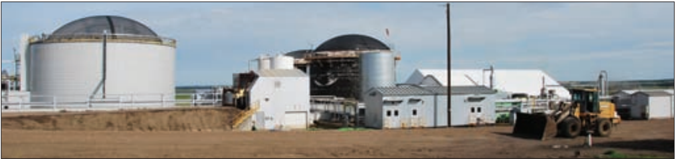
Anaerobic digesters at Highland Feeders Ltd. capture added value from manure, producing 2.5 Mw of electricity. PHOTO BY: MIKE KOTELKO
